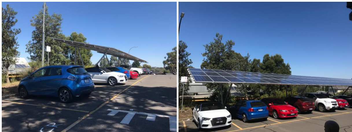
Figure 16: Example of Carpark Solar Panels that can be used for charging infrastructure. Charging EVs with solar generated electricity can result in zero net carbon emissions
