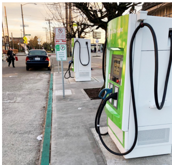
Figure 53 Two DC Fast Chargers owned by Seattle City Light on the 2500 block of 16th Avenue S
