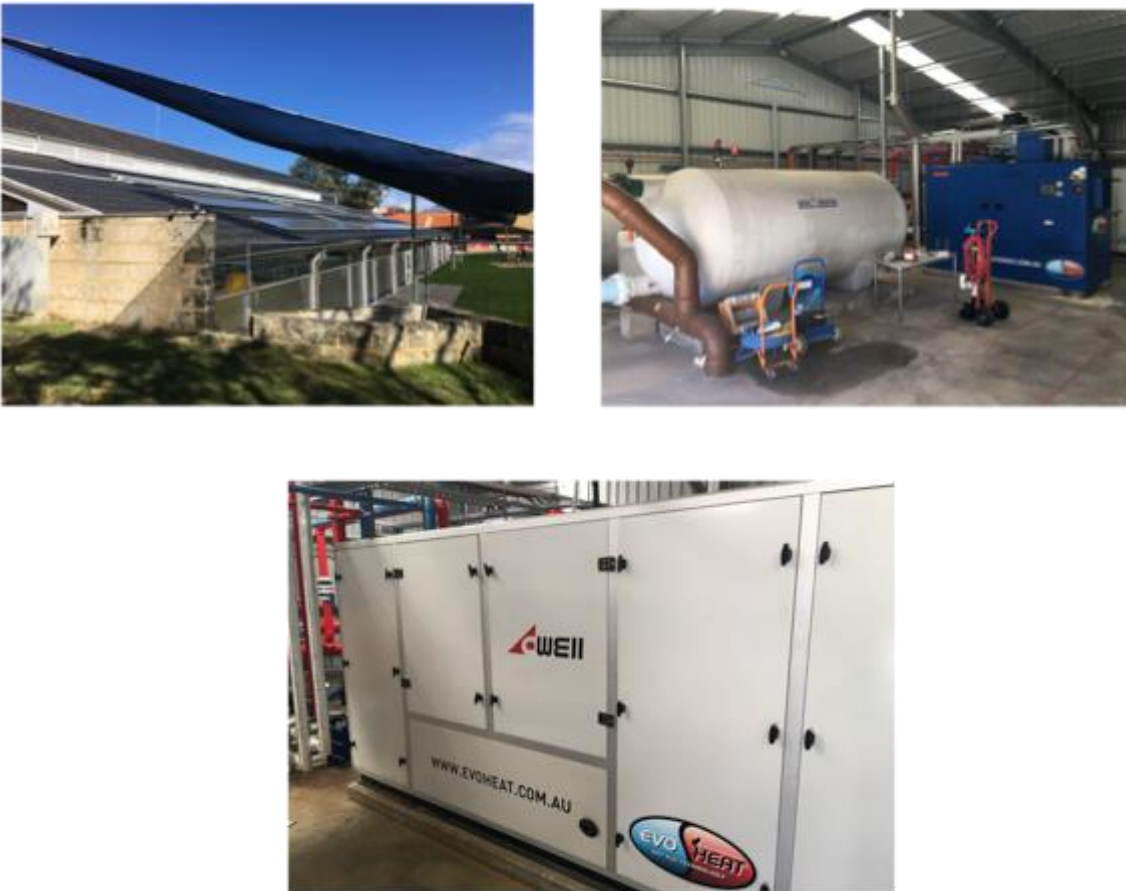
Figure 9: Clockwise from top left: Solar PV panels, the co-generation plant and the geothermal plant.
