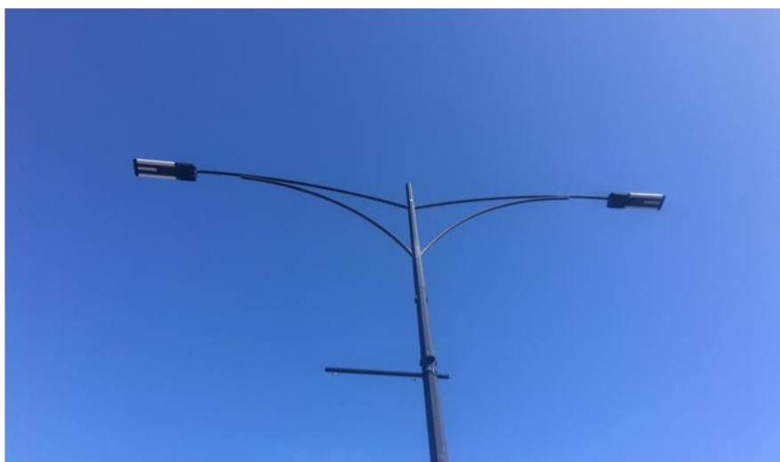
Figure 13: LED streetlights at the Maritime Museum near E-Shed. Installed by the Fremantle Port Authority
