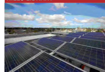
FIGURE 7: SOLAR PV, SURRY HILLS LIBRARY
