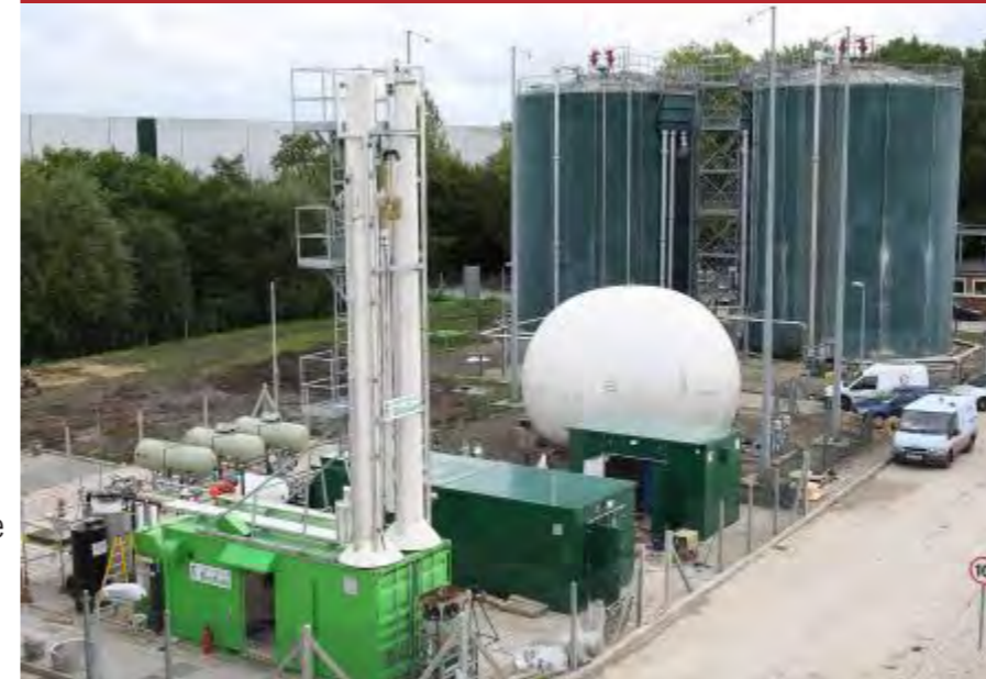
FIGURE 79: DIDCOT SEWAGE TREATMENT PLANT RENEWABLE GAS GRID INJECTION, OXFORDSHIRE, UK SOURCE: CNG SERVICES
