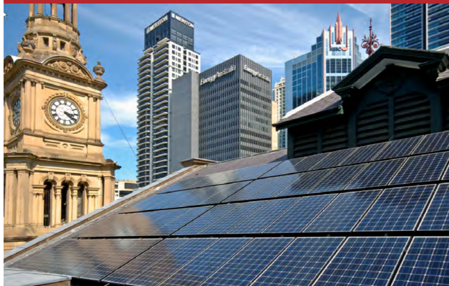
FIGURE 54: SOLAR PHOTOVOLTAIC ROOF SYDNEY TOWN HALL SOURCE: CITY OF SYDNEY
