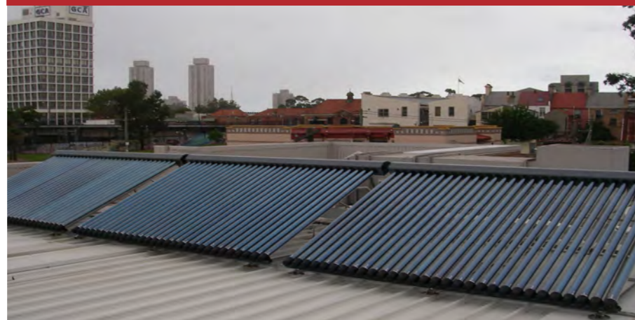
FIGURE 56: SOLAR THERMAL HOT WATER, REDFERN COMMUNITY CENTRE, SYDNEY SOURCE: CITY OF SYDNEY
